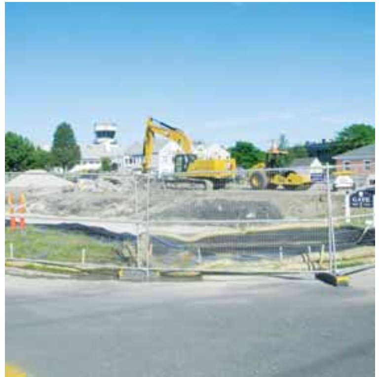
A view of the current construction at the Norwood Memorial Airport parking lot.
