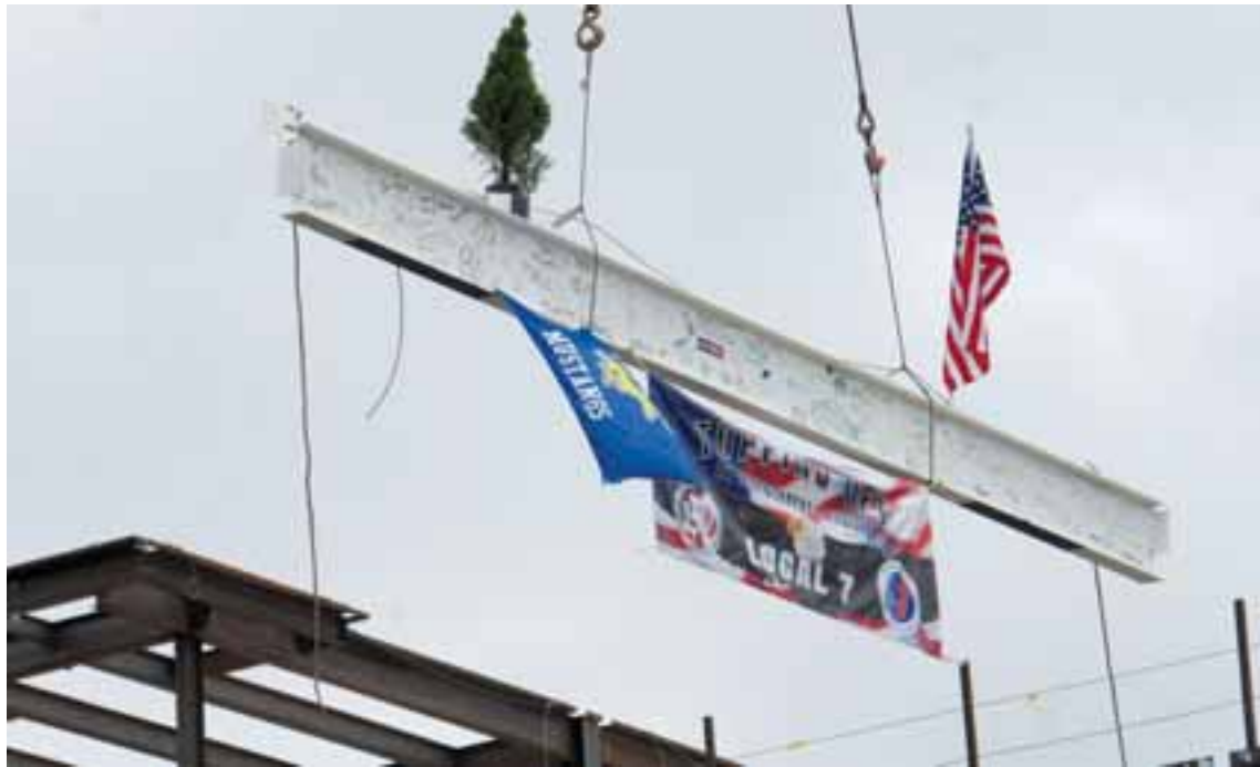
About 100 residents, officials, construction workers and hospital employees came out to sign their names and give the ceremonial girder a send off on Friday last week.
