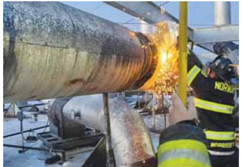
Firefighters worked on the roof to knock down fires that spread to the building’s ventilation system.
