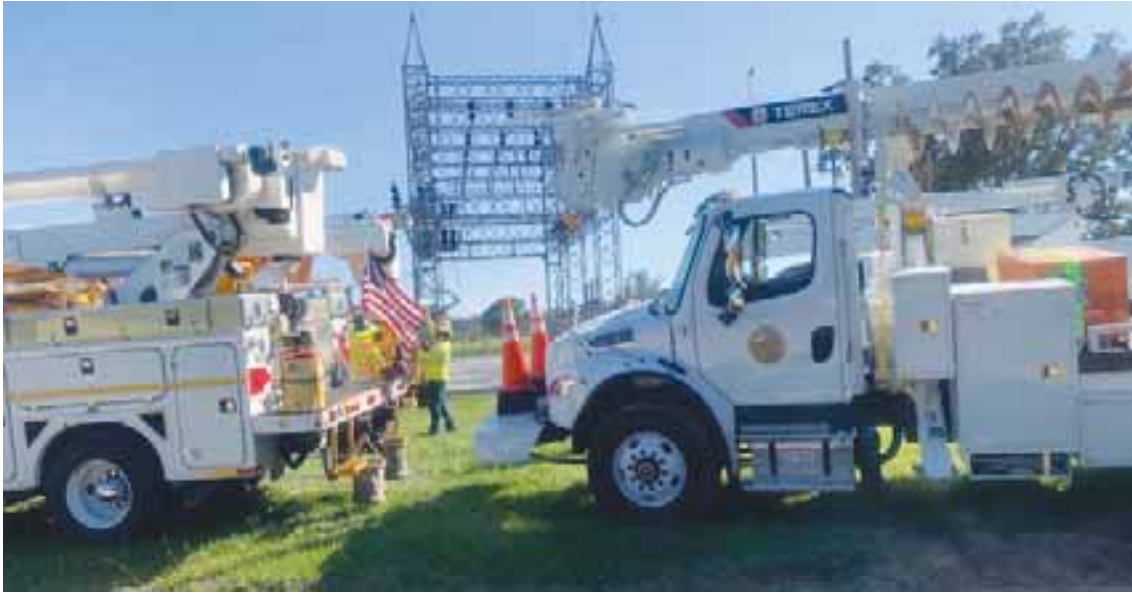
Norwood Light linemen went out last week to help cleanup and power up Jacksonville Florida after Hurricane Ian made landfall.
