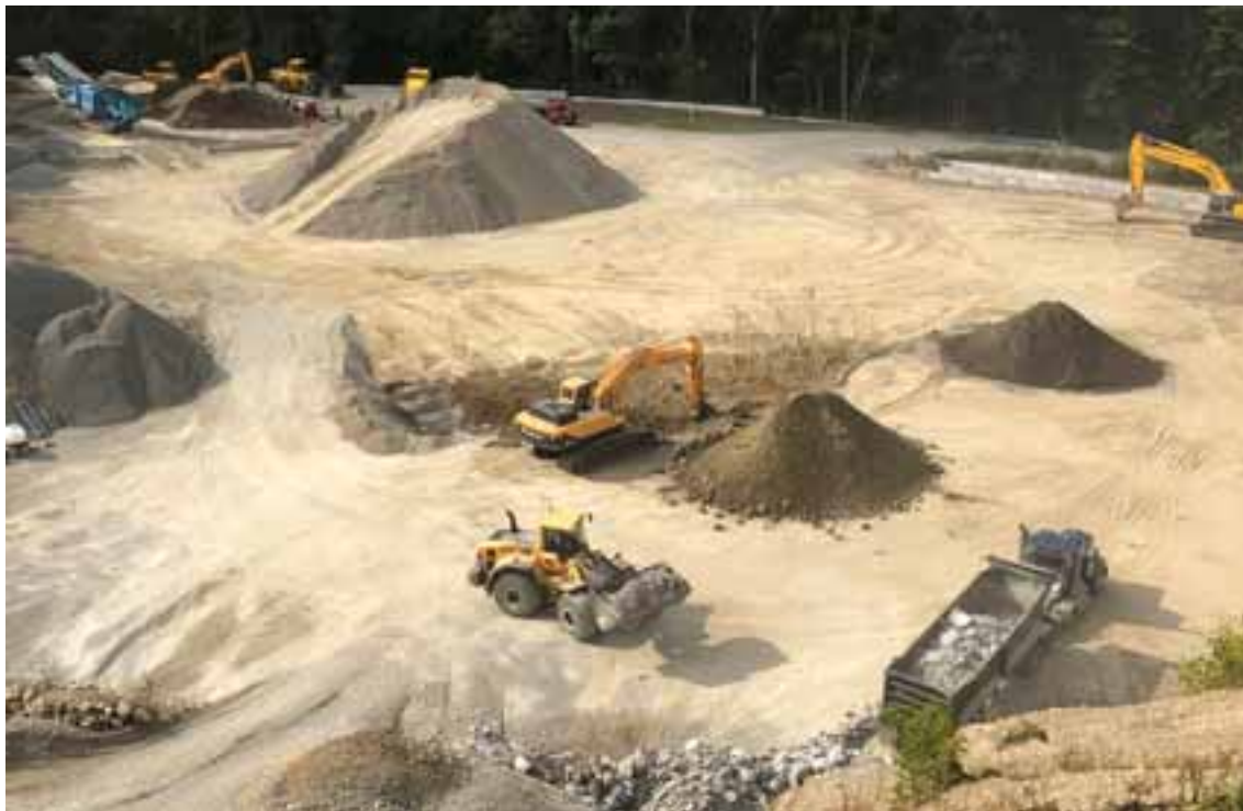
The earth removal site at 973 University Ave. extended its permit for four more years, with some conditions from the Zoning Board of Appeals.
