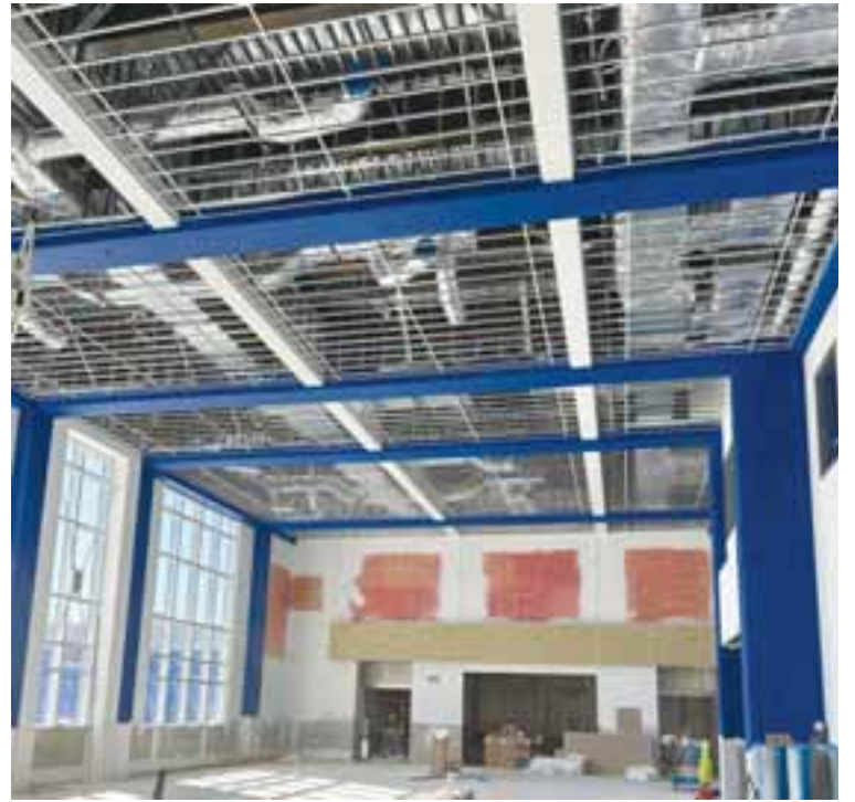
The new mechanical screens would have to be anchored to the building superstructure, shown above, which is why it costs $1 million.
