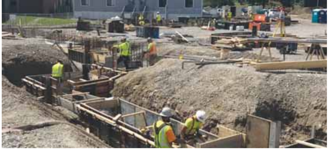
Construction continues at the Coakley Middle School, which could see a name change in the coming weeks, or, it could have residents confirm its current moniker.
