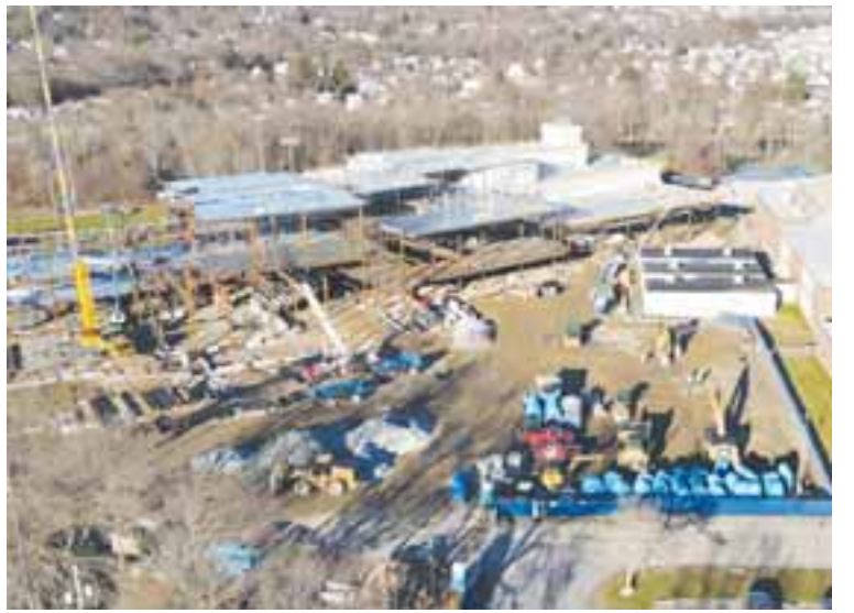
An aerial view of the construction site at the Norwood Coakley Middle School.
