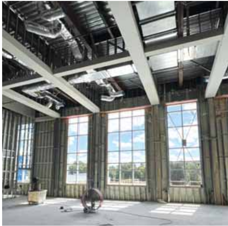
The windows in much of the building are being installed, along with the start of interior work for the building.
