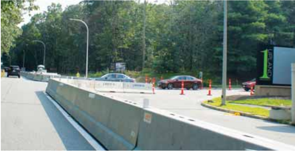
Work has started on Route 1A for a new light at the intersection of Upland Woods Circle and Upland Road. COURTESY PHOTO
