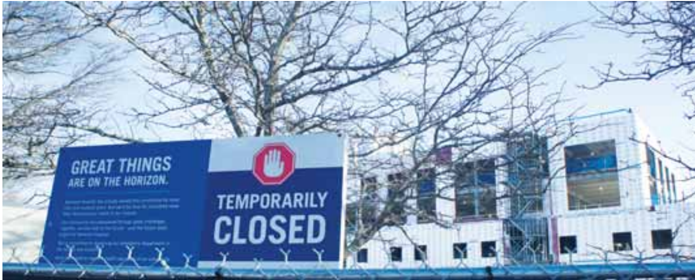
"Great Things" might be on the way, but it is unclear whether it will be Steward bringing them for the new Norwood Hospital.
