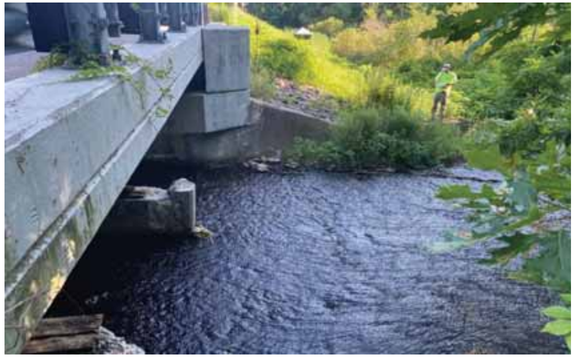
Work will include this spillway on Brook Street, which is in dire need of repairs.
