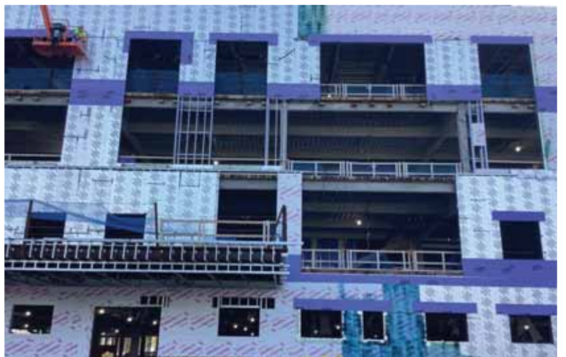
Work continues at the hospital, and windows and the roof are the next major additions on the site.
